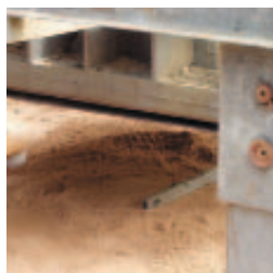
Von Roll blast floor panel BEFORE explosion
